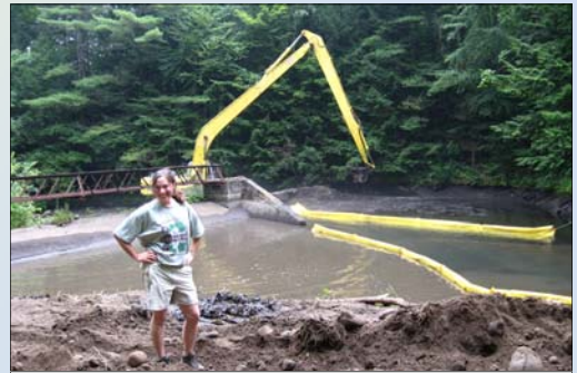
Natural Resources Specialist Lori Kerrigan arranged and managed six reservoir cleanouts in 2009
